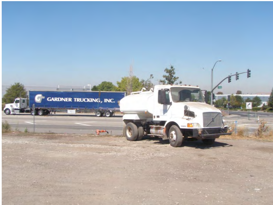
Photo 2: Looking west from access driveway at water truck used for dust control. Water is obtained from the off-site red hydrant located along Greenville Road.
