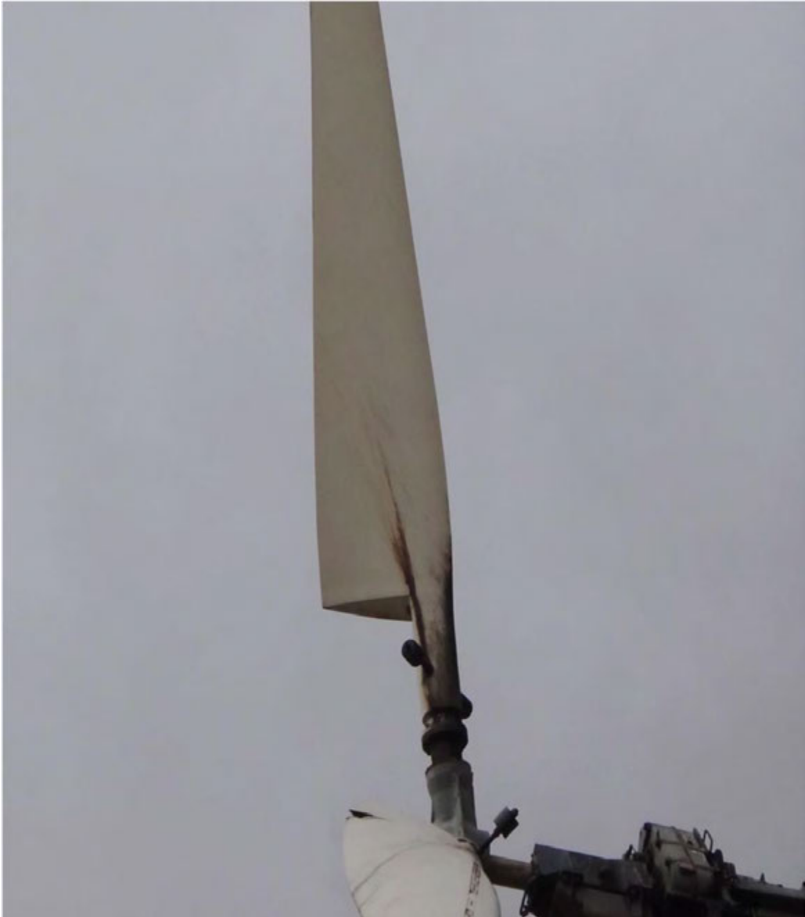
FIGURE 3 CLOSE-UP VIEW OF WIND TURBINE BLADE IFD ROD
